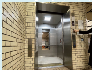
Wheelchair Accessible Elevator
